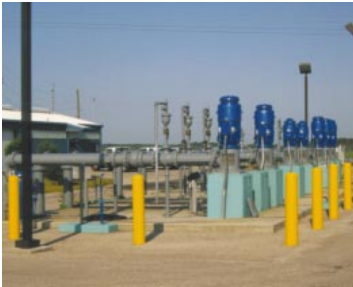
There are 8 pumps that handle all of the irrigation needs for the entire project.
